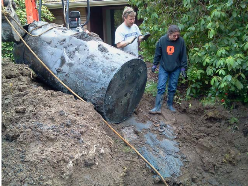
One of three leaking heating oil tanks removed from Kukutali residence site.
