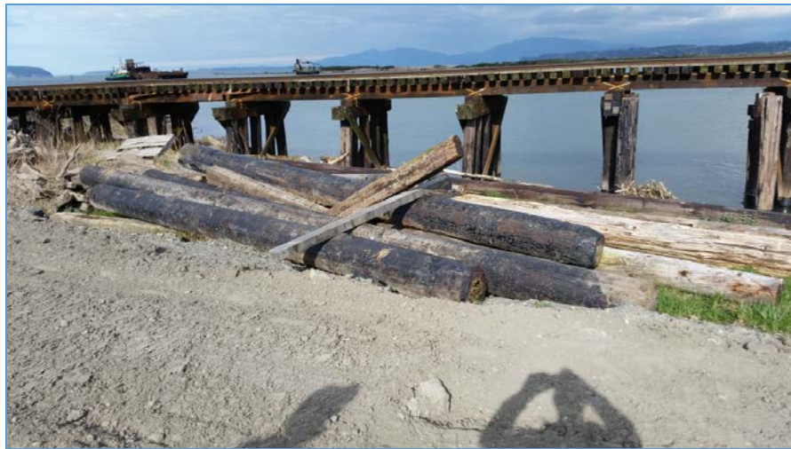
One of two piles of creosote treated debris removed from the vicinity of the Swinomish dock (TEZ area 1) in 2015
